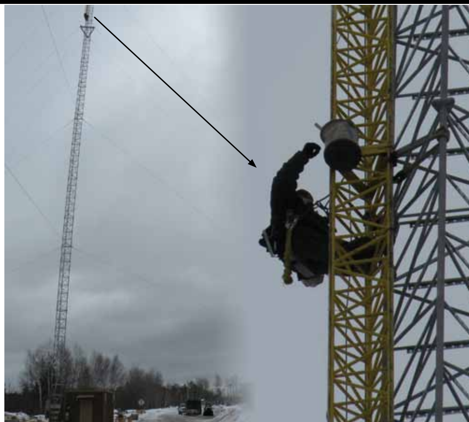
A worker installs the one of the top sections of the 500 foot radio tower. The tower was completed on February 16th, 2011
